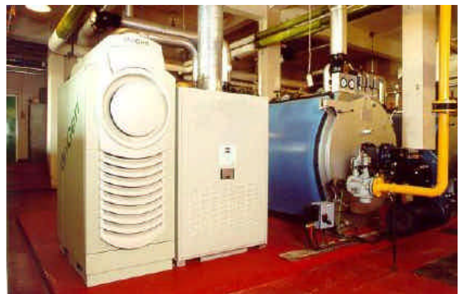
Figure 16. A 30-kW microturbine provides heat and power for a municipal building in Durham, England. Photo courtesy of Capstone
