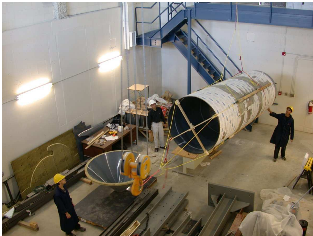
Figure B.4: Two cranes lift the reaction chamber up and then orient it vertically to be dropped on to the support structure. The cone, resting on the ground, is also visible.
